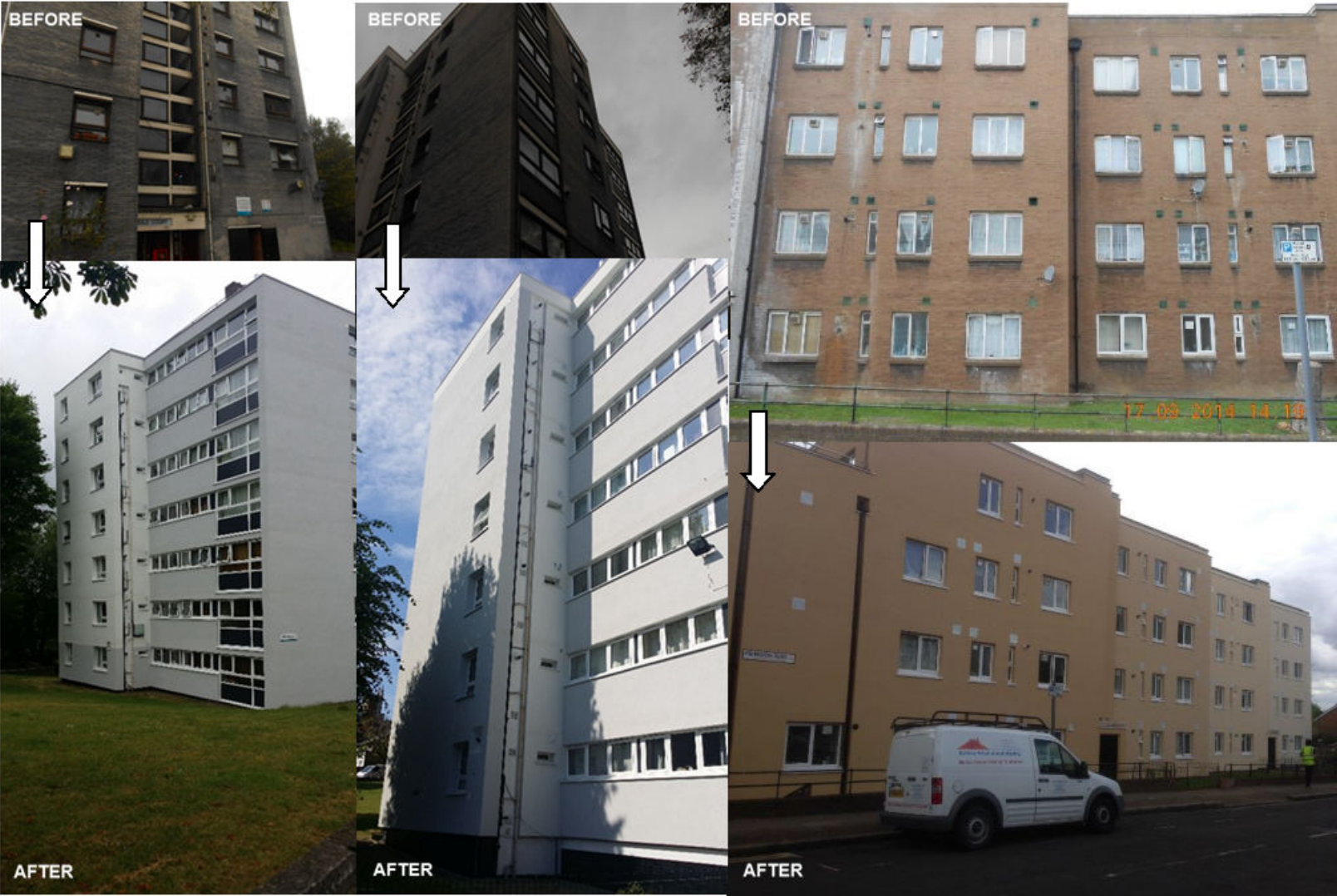
Forbes, Gould and Heaton House—before and after (In Partnership with A&E Elkins)
